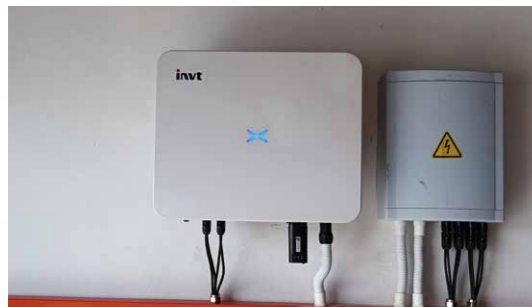
25kW Solar System in Malaysia (XG25KTR)
