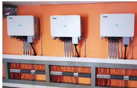
180kW Rooftop PV Plant in Lebanon (XG60KTR)
