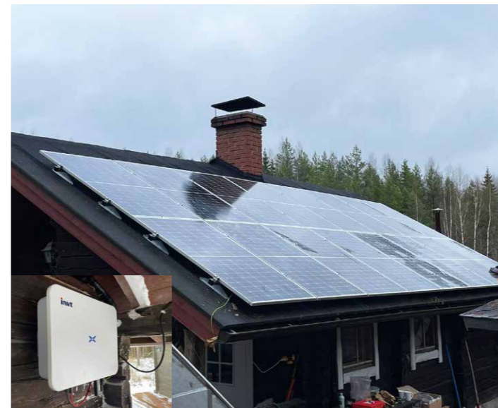
8kW Solar System in Finland (XG8KTR)
