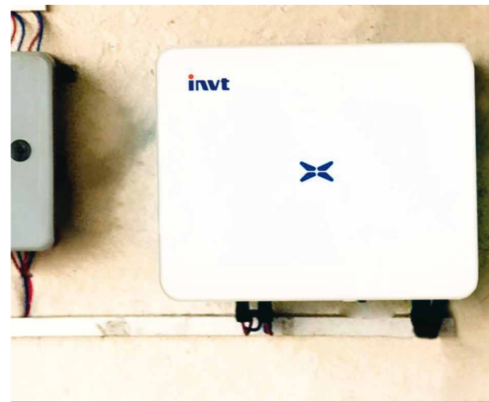
10kW Solar System in Armenia (XG10KTR)
