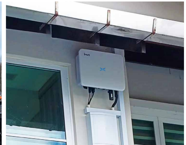
12kW Solar System in Malaysia (XG12KTR)
