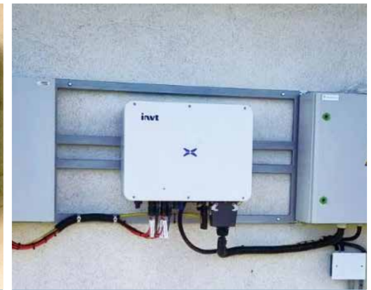
30kW Solar System in Serbia (XG30KTR)
