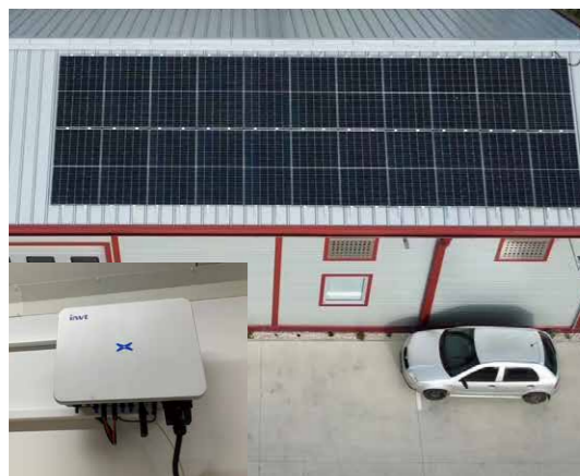
25kW Solar System in Slovakia (XG25KTR)
