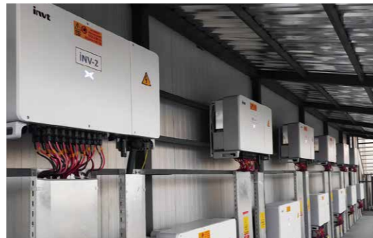
2MW Rooftop PV Plant in Türkiye (XG110KTR)
