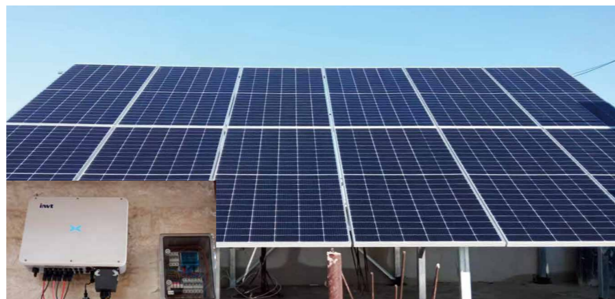
30kW Solar System in Israel (XG30KTR)
